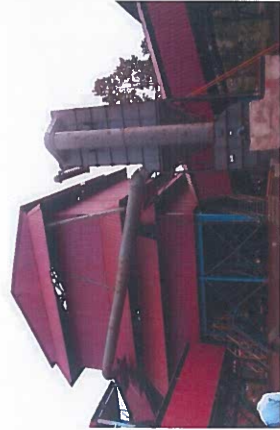
Photo – 15 showing the Screening plant equipped with bag filter system & dry fog system
